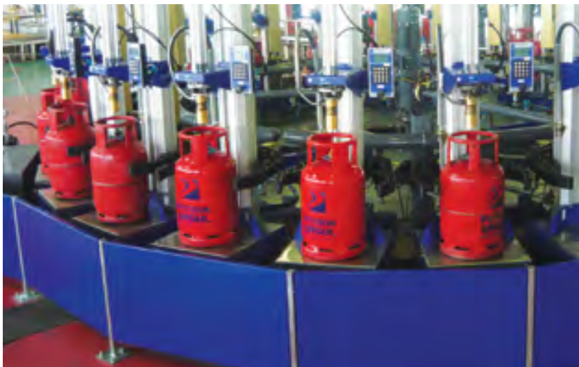
Newly installed LPG filling machine at PDT to support growing demand
