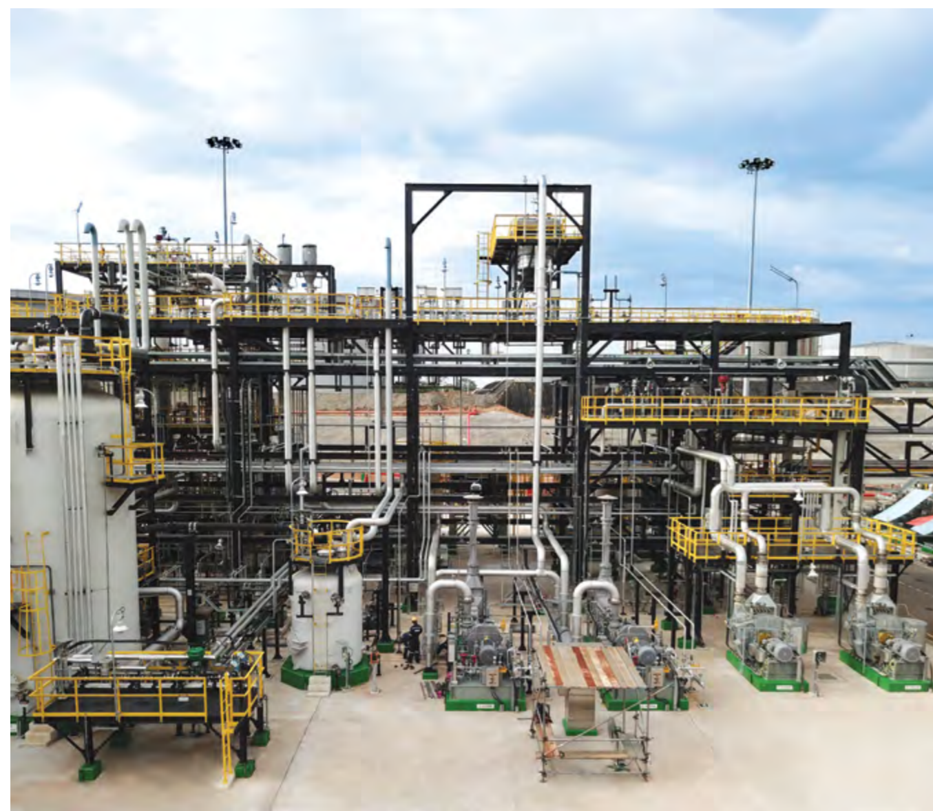
● Port Dickson Refinery Diesel Hydrotreater is the newest facility to produce low sulphur diesel, Euro 5.
